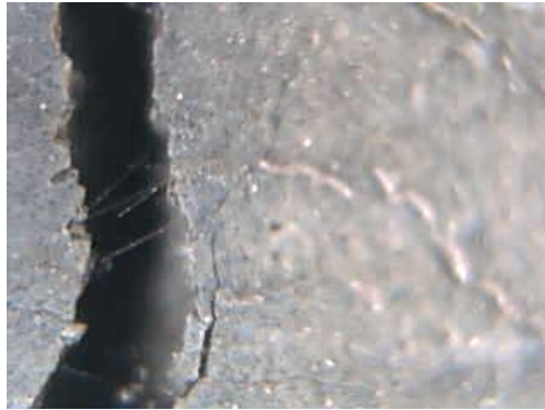
Figure 1: Partial enlarged photo of fiber concrete
