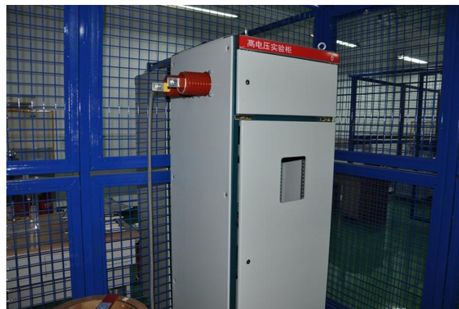
Figure 1: 10kV switchgear for experiment
