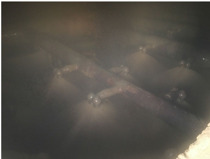
Figure 2. Photo of Nozzle Condition
