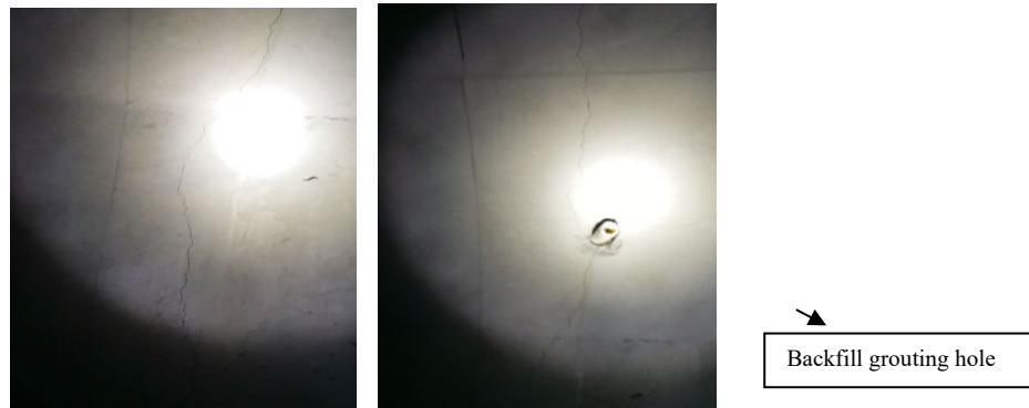
Figure 1: Cracks of the side wall Figure 2: Cracks of the vault
