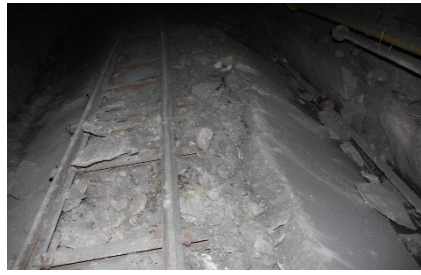
Figure 1: Deformation and Failure of Rail Track Crosscut
