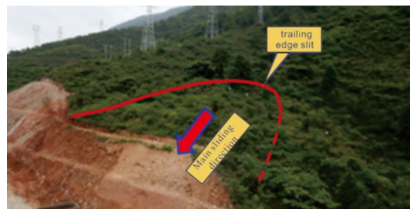
Figure 1: Landslide on the right of CK0 + 820~CK1 + 000 of Songkan Hub
