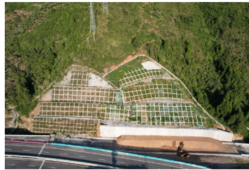
Figure 2: Landslide on the right side of CK0 + 820~CK1 + 000 section of Songkan Hub interchange
