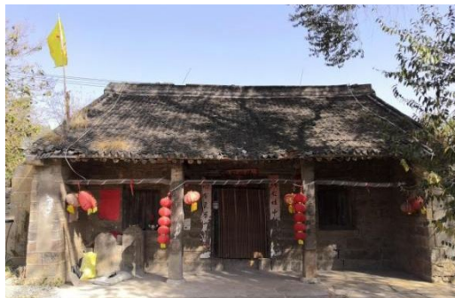
Figure 4: Residential houses with too long eaves
