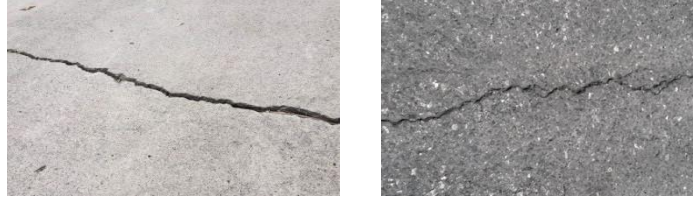
Fig.1 Pavement Crack Map
