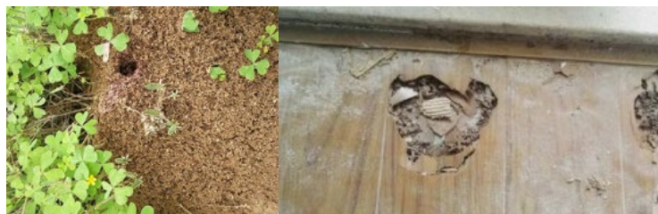
Figure 1 Damage caused by termite infestation
