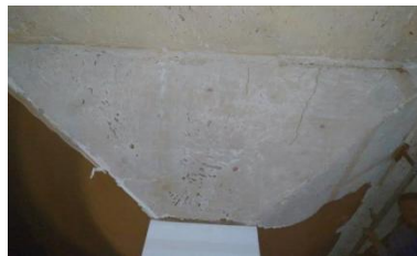
Figure 2: Photos of vertical cracks in column caps
