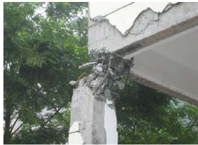
Figure. 3 Shear failure of corner column of frame structure
