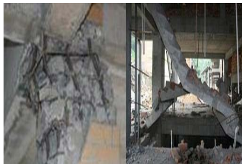
Figure. 2 Frame node failure
