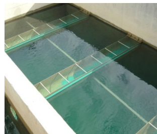
Figure 5: Filtration facility at McAllen Northwest [16]
