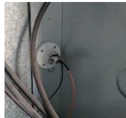
(c) TEV sensor installation.
