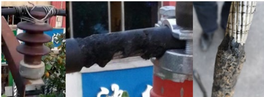
Figure 1: Partial Discharge Problem and Burned Insulation on Covered Conductors.
