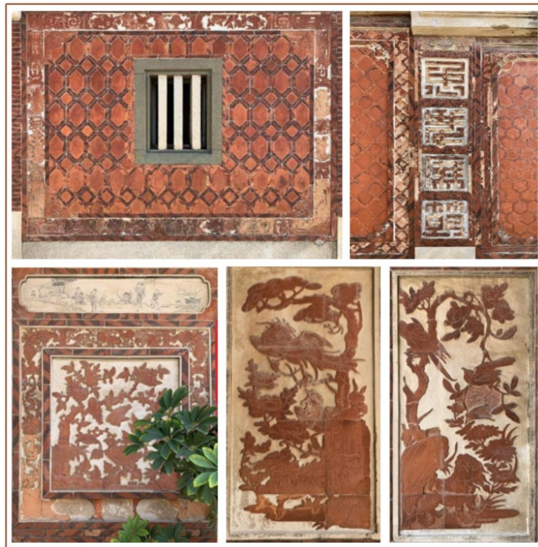
Figure 2: The Weathering Status of Brick Carving
