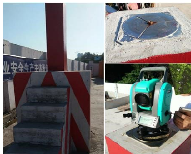
Figure 2. Schematic diagram of site monitoring and measuring point layout of bridge pier
