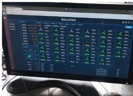
Figure 7: Wind turbine host computer monitoring system.
