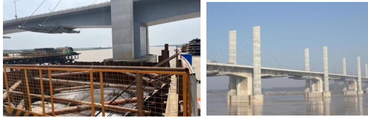
Figure 1: Schematic diagram of the reinforced cable-stayed system and deep foundation pit of the main bridge of Dongming Huanghe River Bridge.
