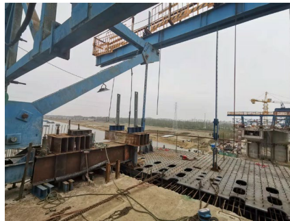
Figure 7: Site photos of the hanging basket and temporary hoisting and fixation device
