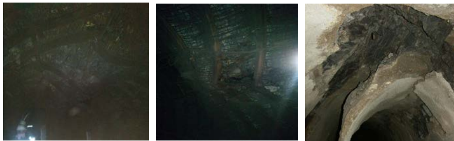
Fig.2 Deformation and failure characteristics of surrounding rock
