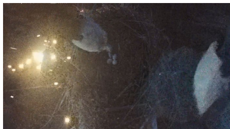
Figure 3: Flashover fault caused by Oriental white stork's droppings in the early morning in Daqing area
